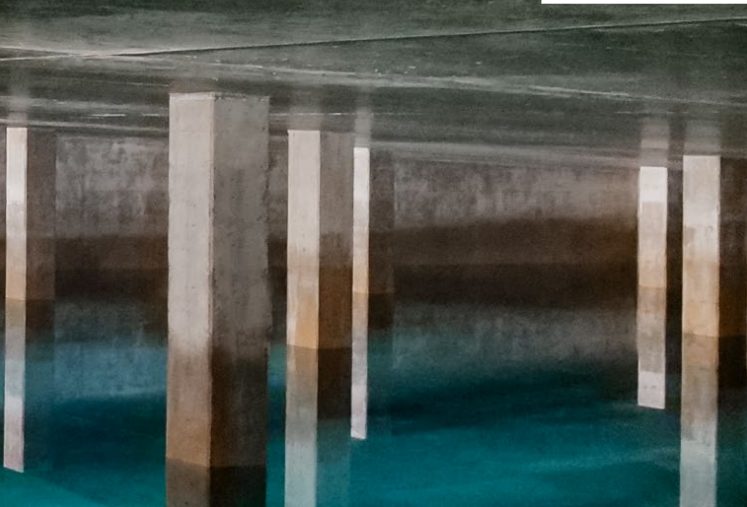
The ZUG LED luminaires with their lens-type appearance and an emergency luminaire with a tube consisting of clear PMMA and potting are precisely adapted to the conditions in the water storage tank.
