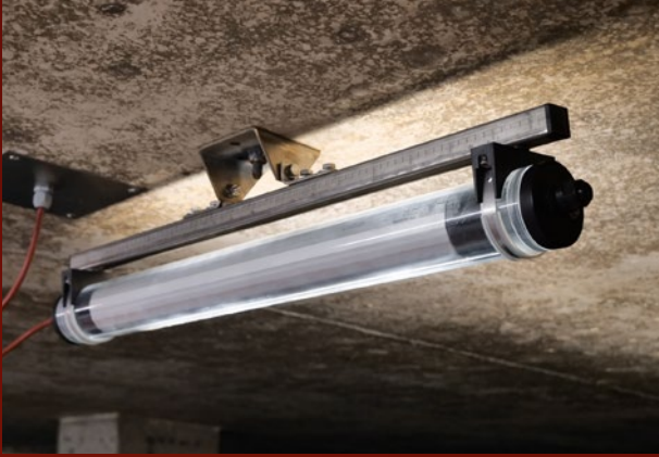
> Project version ZUG LED with lens technology and moulded connection cable
